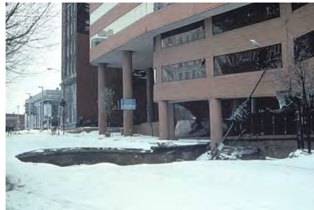
Sinkhole at Corporate Plaza Building in Allentown, Lehigh County, PA in February, 1994 (Photograph by William E. Kochanov . PADCNR, 2009).
