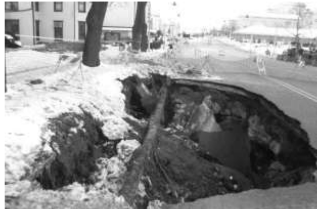
Sinkhole in Dauphin County has exposed a utility pipeline ( Kochanov , 1999).
